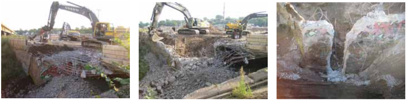
Figure 4: Careful demolition of the bridge revealed the reinforcement, facilitating its documentation in selected areas.
