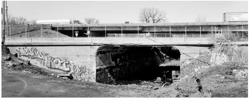
Figure 1: Bridge No. 92297 shortly before demolition. Photograph by Daniel R. Pratt, courtesy of MN Historical Society Archives.
