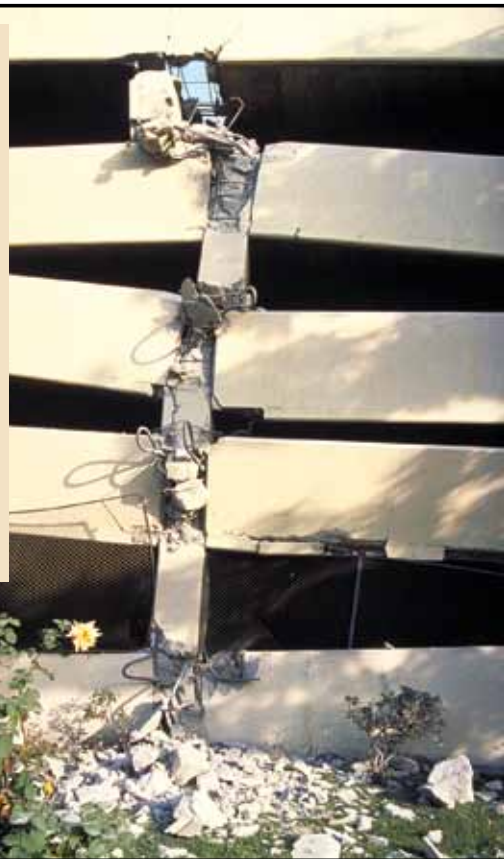
Figure 1: Collapsed parking structure, 1994 Northridge Earthquake. Courtesy of Robert Reitherman.
