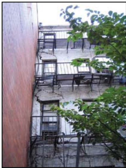
Figure 5: Damage resulting from adjacent construction.
