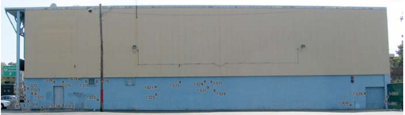
A photo of a building elevation can be used as a key map for identification of individual distress, shown separately on detailed, up-close photos.
