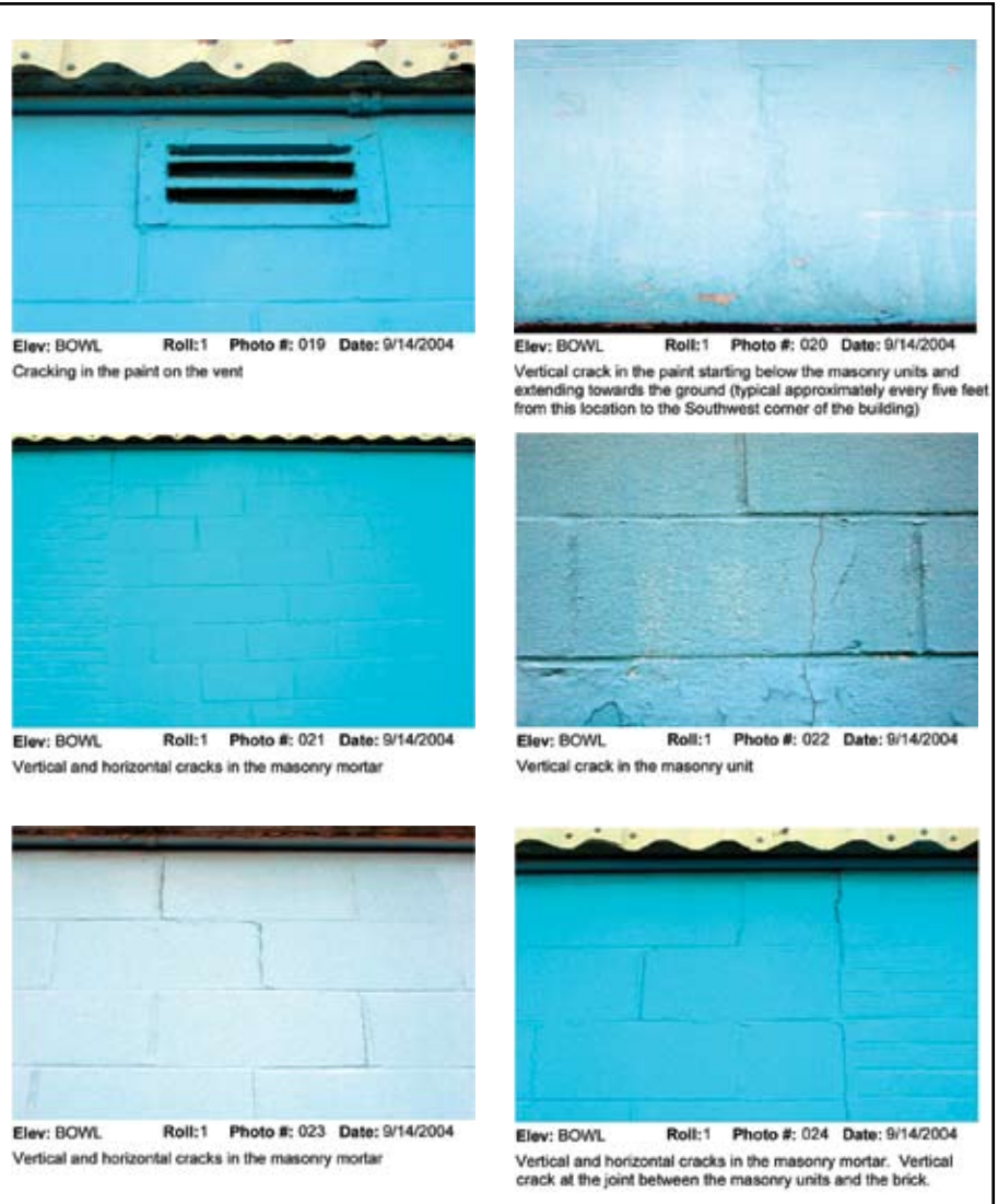
Detailed observations from a condition survey can be shown on individual photos linked to a key plan.
