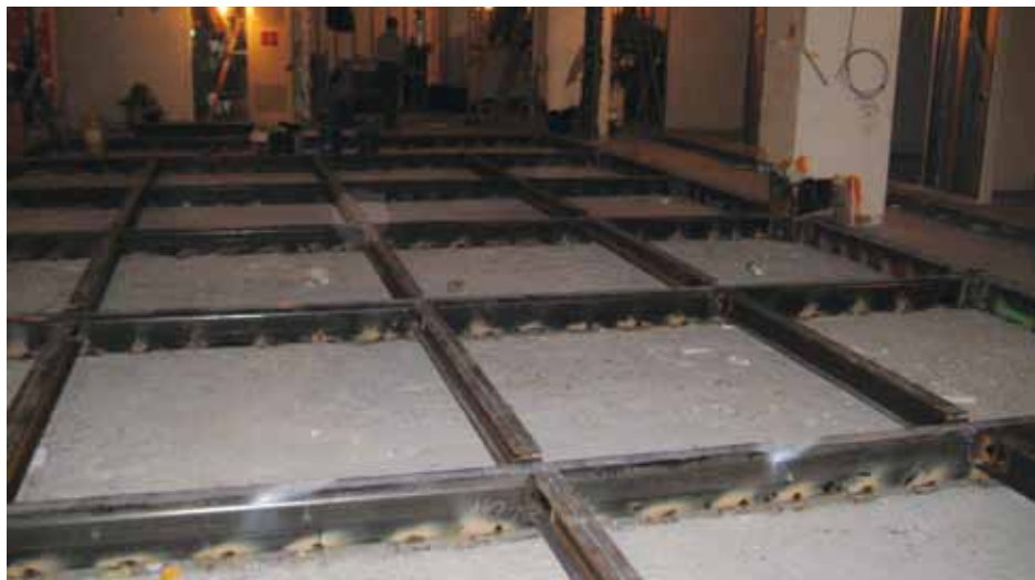
Figure 4: (Structural analysis and design) When existing structural elements are inadequate, and access is not available, unique solutions are required. Here, designers trenched the concrete fill at the steel beams and welded tubes to their top flanges. Then a framework of filler beams was created that would support the track loads from the high-density file system. All beam topsides and tubes were hidden in a raised floor system.
