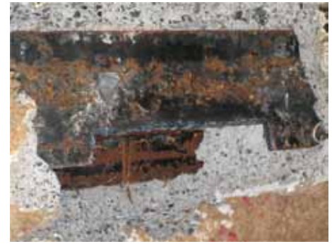
Figure 2: (Field investigation) Removal of finishes, concrete coring and other testing can reinforce available shop drawings and confirm structural details.
