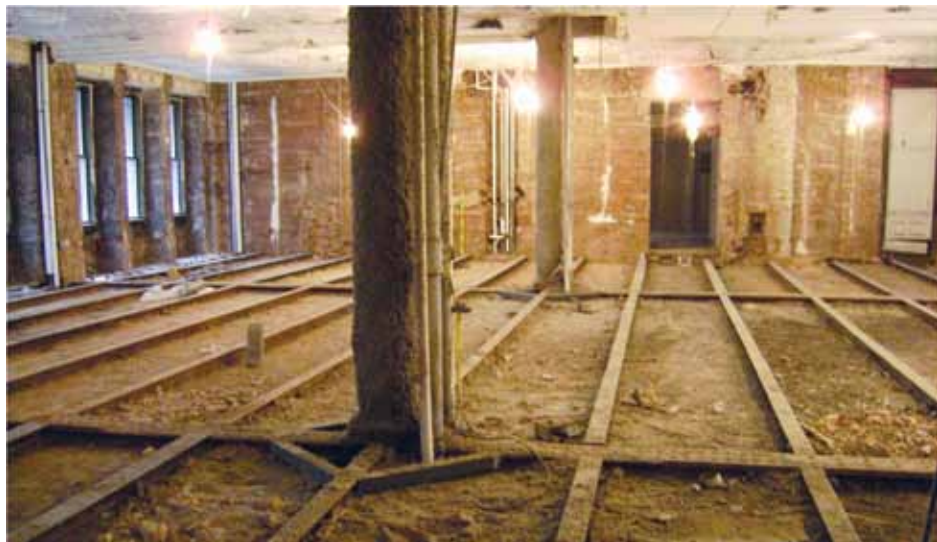
Figure 3: (Field investigation) In some instances, removals allow for new installations. Portions may not require removal, and ground-penetrating radar (GPR) can supply needed information.
