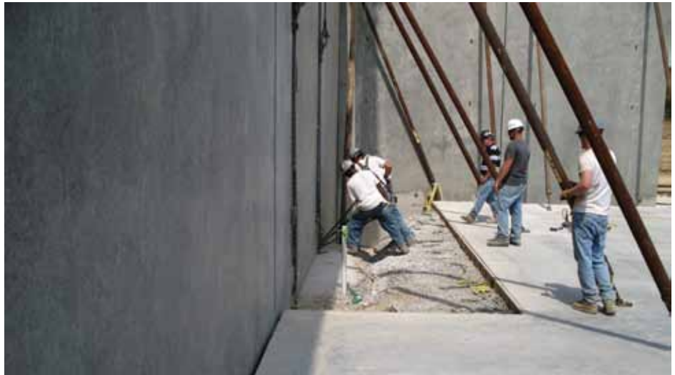
The panel erection crew using pry bars to position the panel into the proper location on the footing.
