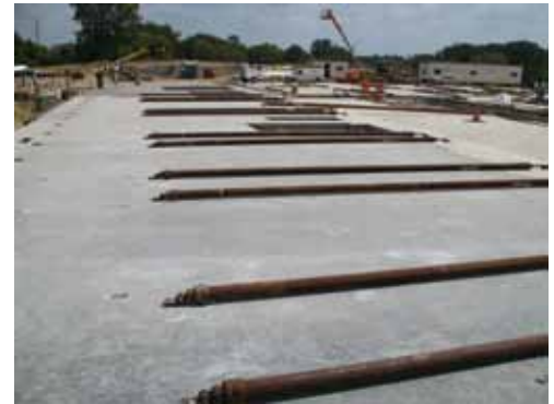
Wall panel temporary braces attached to the inside face of wall prior to panel erection.
