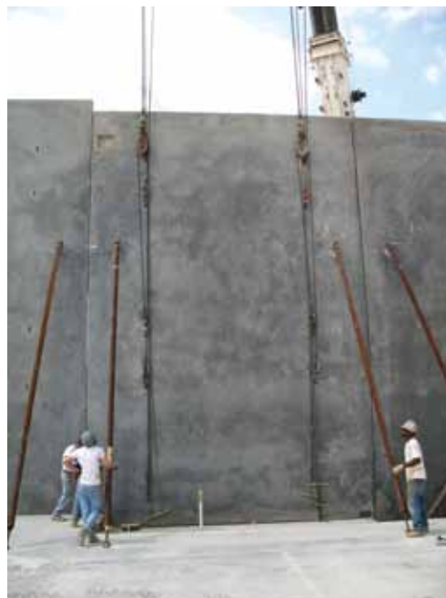
The panel erection crew winding the temporary braces for final plumbing of the wall panel during erection.
