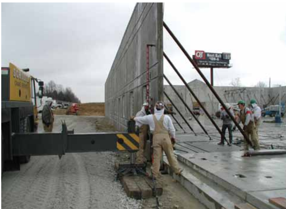
The panel erection crew using an extendable level to check plumb of the wall panel.
