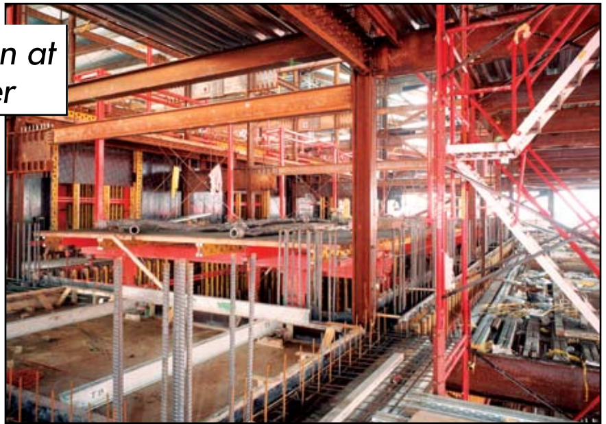
Automatic Climbing System Unit being Raised Through Steel-framed Skeleton in Building Core. Courtesy of Austin Gelbard (Tishman Construction).
