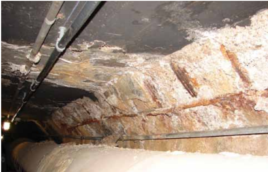
Figure 2. Corrosion damage in tunnel section.
