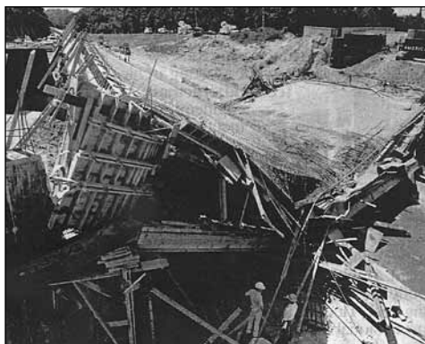
Figure 9: Baltimore-Washington Parkway. End view of collapsed falsework. (From ENR, September 7, 1989)
