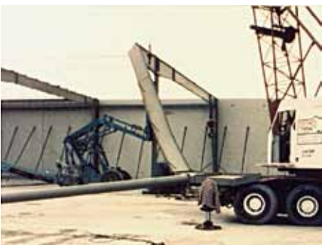
Figure 6: Toppled column during erection.
