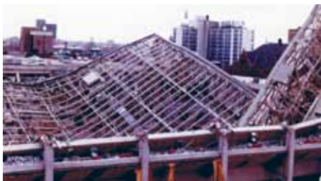
Figure 1: Collapsed space frame roof at Hartford Civic Center.
