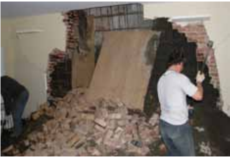
Figure 5: Collapsed wall adjacent to construction site.
