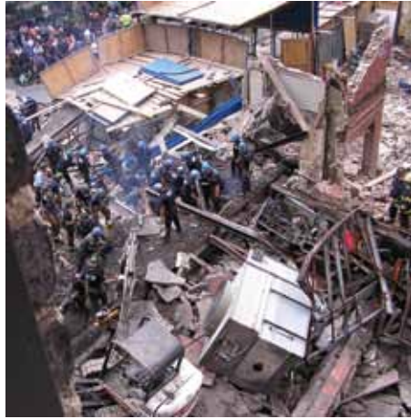
Figure 7: Collapsed building during demolition.
