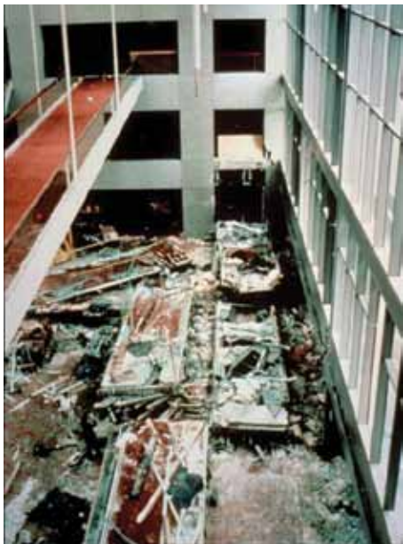
Figure 2: Collapsed skyways in Kansas City Hyatt Hotel.
