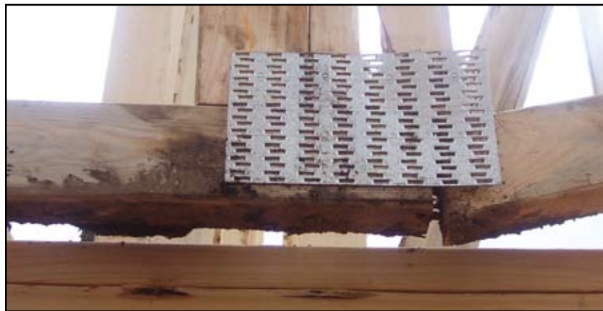
Figure 1: A typical damaged joint. Notice the connector plate teeth have pulled out of the lumber on the right side of the joint, and one web is split along the grain. Also, note the mud on the lumber, a consideration when using adhesives.
