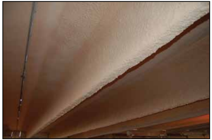
Figure 6: Parking Garage (rare inclined cracks).
