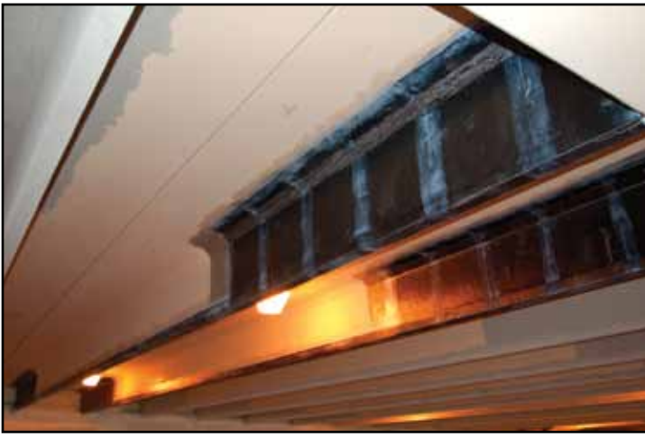
Figure 5: Parking Garage (rare inclined cracks).
