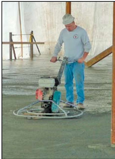
Figure 6: Finisher making first pass over lightweight concrete with walk behind power trowel.
