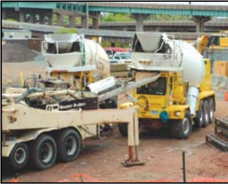
Figure 4: The concrete pump should have access for two ready mix trucks to prevent delays in pumping.
