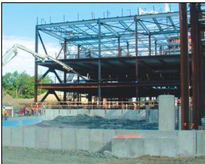
Figure 2: Most of the structural lightweight concrete that is placed in commercial structures is pumped.
