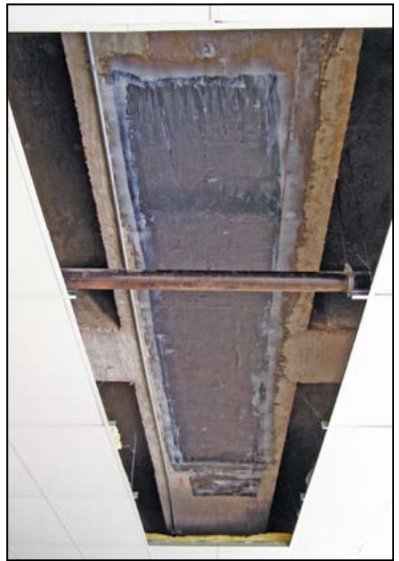
Carbon-based FRP installation on the soffit of an existing beam. Courtesy of Walter P Moore.
