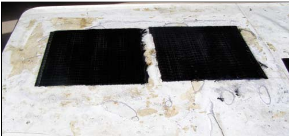
An example of a carbon-based FRP witness panel prepared in the field for laboratory tensile testing. Courtesy of Walter P Moore.
