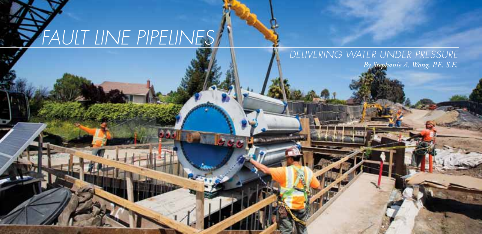
Figure 1. The slip joint was lowered into the vault by crane. Courtesy of San Francisco Public Utilities Commission, Robin Scheswohl.
