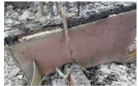
Figure 4. View showing the characteristic pink hue of heat-damaged concrete. The signature pink color is a strong indicator the concrete is severely damaged and cannot be re-used for reconstruction.
