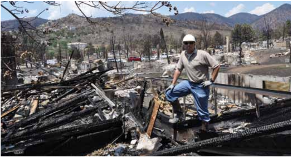
Figure 1. View showing the widespread damage that occurred through this suburban neighborhood following the Waldo Canyon fire.
