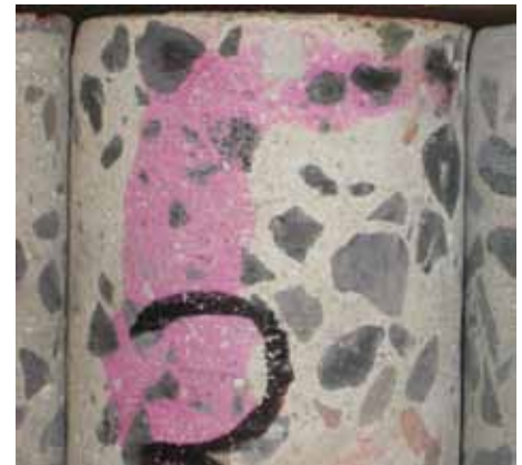
Carbonation Test Results at a Concrete Core Sample.
