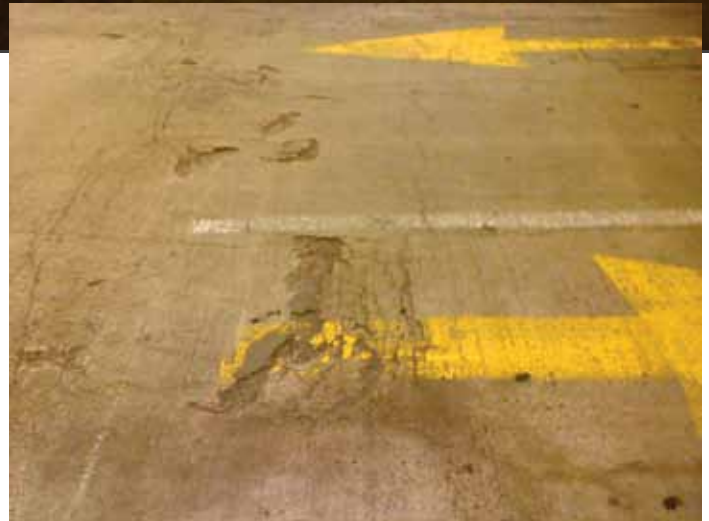
Typical Surface Spalling and Cracking.
