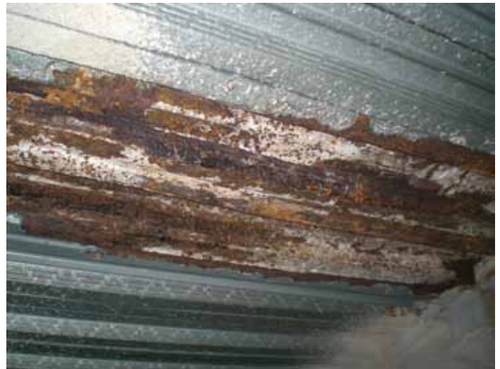
Typical Composite Metal Deck Corrosion.
