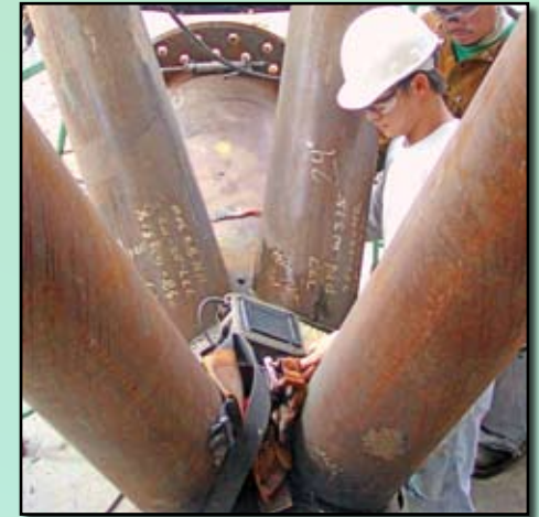
Figure 4: A certified inspector checks out full penetration welds of diagonals on bottom-pipe saddle while the welder looks on
