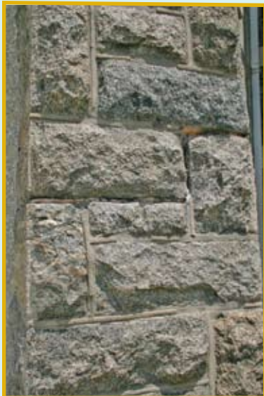
Figure 1: The inspection identified a need for a great deal of tuck pointing on the masonry.
