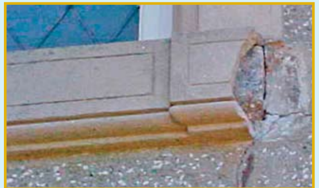
Figure 3: Significant patching was necessary for the limestone.
