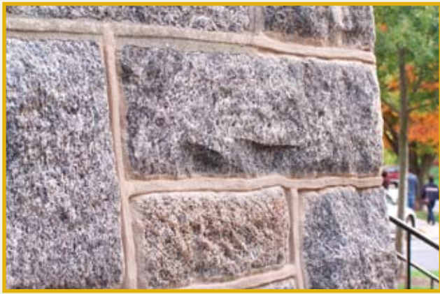
Figure 7: Several mortar samples were made in order to find the right color mix for the deteriorated mortar ribbon joints and the random joints needing re-pointing.
