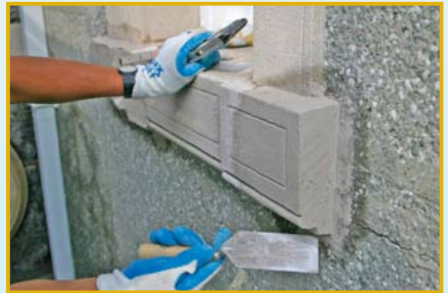
Figure 6: The spalled and deteriorated areas of ornamental stucco detail were repaired using a premium grade stone repair mortar.
