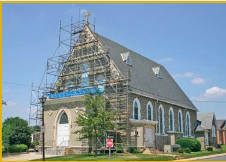
Figure 5: Scaffolding was erected at the main entrance to the church in a manner that still allowed access to the structure during the work week
