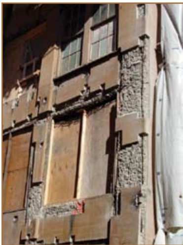
Figure 2: Close up view of the prepared concrete in the South elevation. Removal depths of three inches were commonplace.
