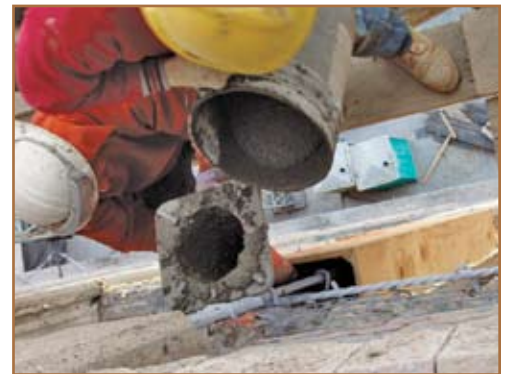
Figure 3: Workers placing the cementitious repair mortar via form and pour methodology into a sealed plywood form.
