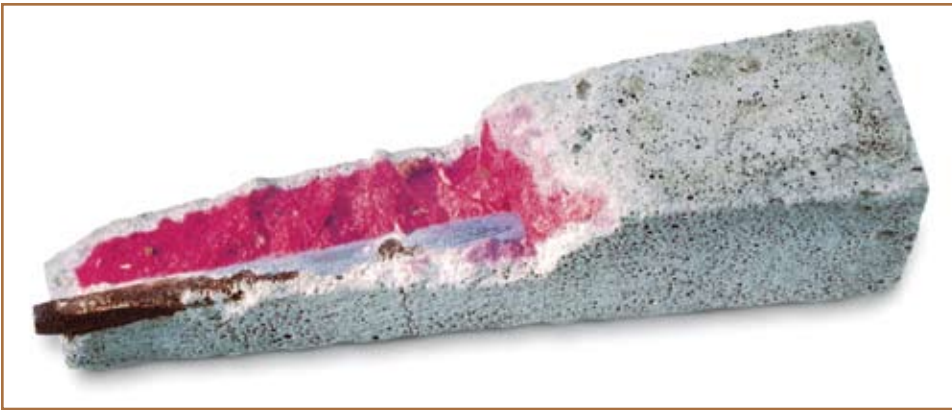
Figure 4: Photo showing the chemical reaction of phenolphthalein with an alkaline environment and it clearly identifies the presence of a “carbonation front”.
