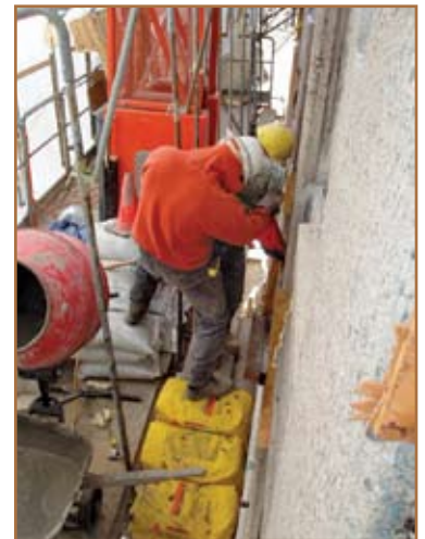
Figure 5: Contractors set up including repair mortar, bagged stone, electric mixer and wheelbarrow.
