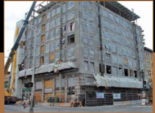
Figure 1: The North and East elevations with the extent of the façade repairs.
