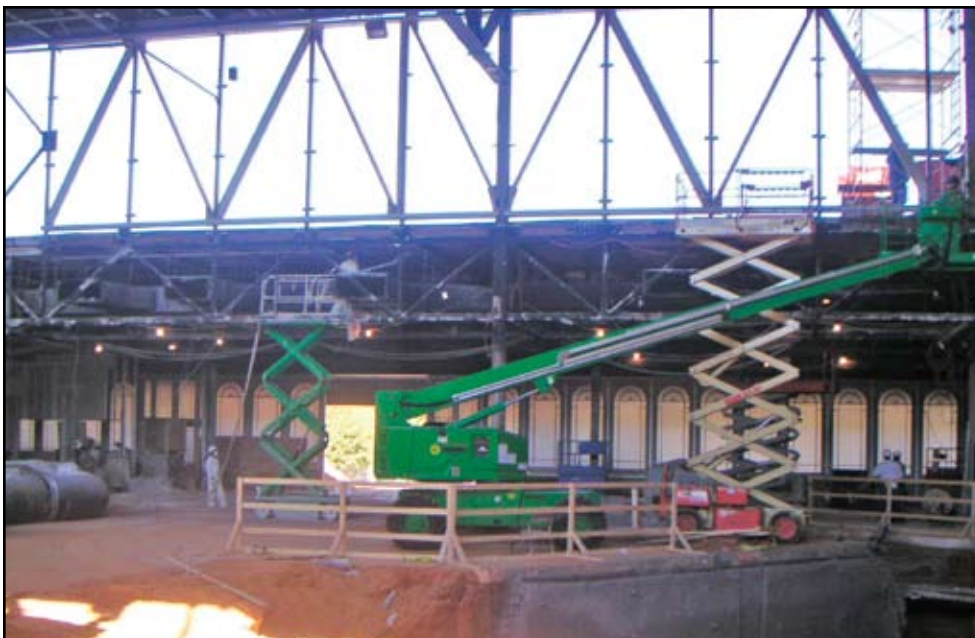
The new truss that was added between the low roof and the high roof, using the existing post as part of the truss.
