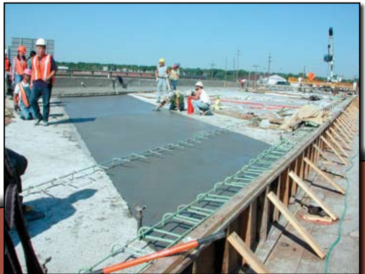
Figure 3a: Completed ECC Link-Slab (Phase 1) on the Grove Street Bridge in Ypsilanti, Michigan
