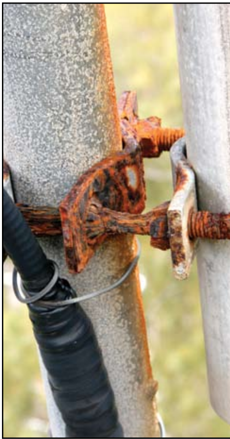
Severe Corrosion on a Tower in Hawaii
