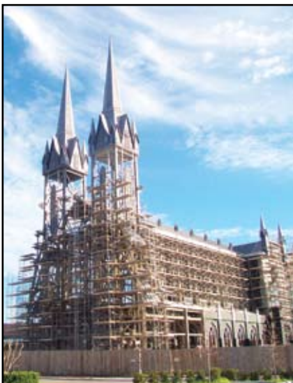
The proximity of the church to occupied buildings and the tight site presented challenges to the design and construction team. Photo by Christof Spieler, P.E.
