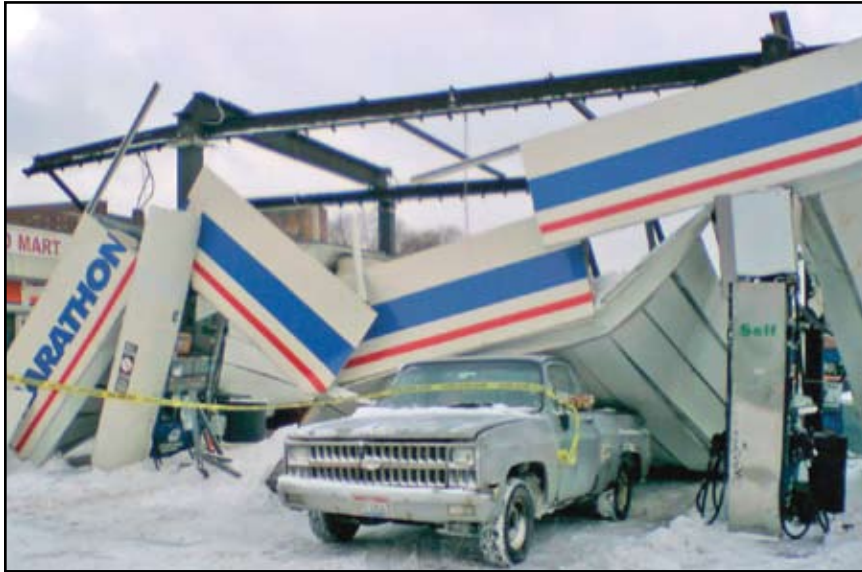
Snow related canopy failure in Cleveland Ohio during the winter of 2006/2007. Courtesy of WKYC.com.
