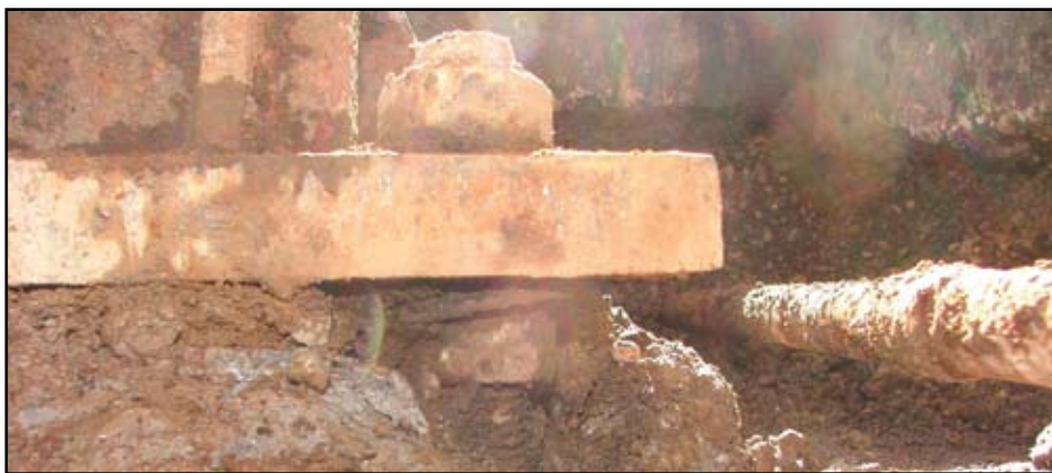
Anchor bolts and washer are being pulled through oversized holes in the baseplate, causing the canopy to lean.
