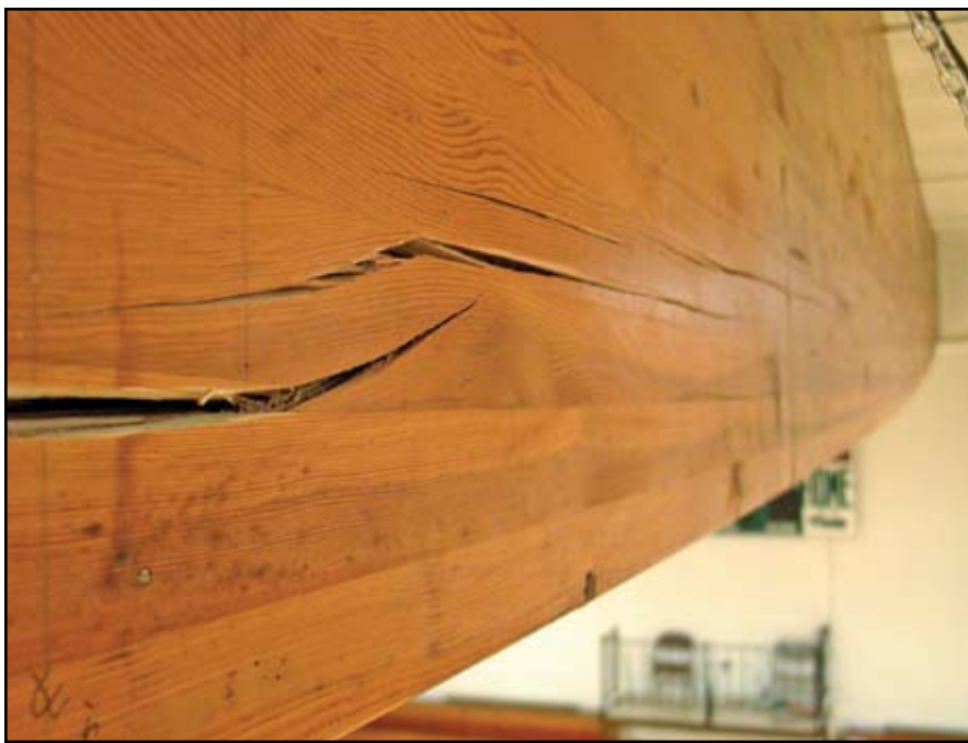
Figure 2: Failed beam due to overstress in bending
