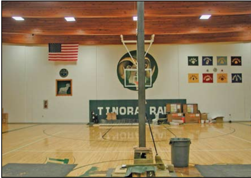
Figure 4: 6 x 6 HSS member used to jack beam to unloaded position during beam repair
