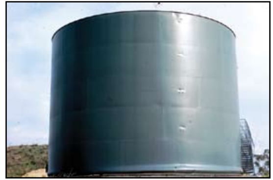
Figure 3: "Elephant Foot" caused by the movement of water in a large steel storage tank during San Fernando, California, Earthquake February 1971. (Courtesy of USGS Photographic library)
