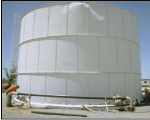
Figure 4: Buckled water tank lifted off base by Landers Earthquake. (Courtesy of Lindie Brewer, U.S. Geological Survey)
