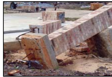
Masonry piers and footings overturned and toppled.
