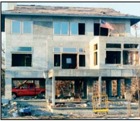
The Sundberg home. Open foundation constructed with reinforced concrete columns and grade beams/footings. Foundation survived even after the home was inundated with six feet of water and exposed to breaking waves and flood-borne debris.
