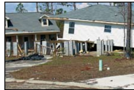
Connection failures allowed homes to float off their foundations.
