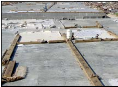
House washed away from its foundation. Only the sill plates remained.
