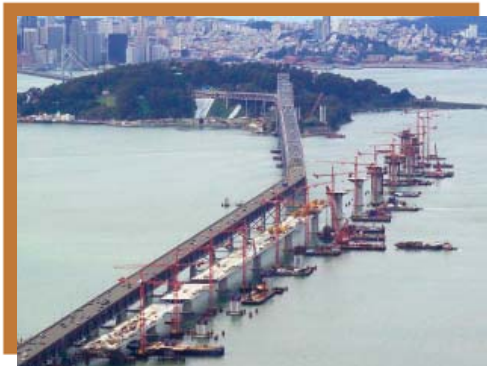
Figure 1: San Francisco-Oakland East Bay Skyway Bridge Construction. Photo courtesy of Kiewit/Flatiron/Manson, A Joint Venture.
