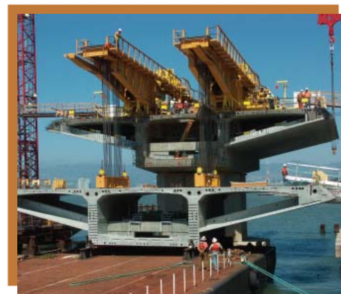
Figure 10: San Francisco-Oakland East Bay Skyway Bridge Segment Erection Device. Photo courtesy of Kiewit/Flatiron/Manson, A Joint Venture.
