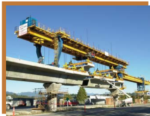
Figure 9: Articulated Erection Gantry for use on Curved Alignment. Skytrain Millenium Line, Vancouver, British Columbia.
