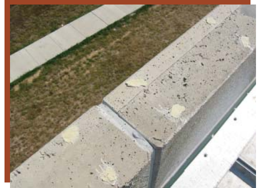
Figure 23: Always use a cap flashing at the top of panel- It's missing here
