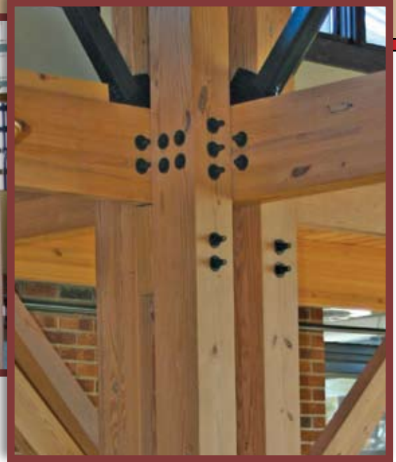
Figure 4: Glulam members were connected using steel plates and conventional split rings. The column clusters allowed efficient "sandwiched" connections to load the carrying trusses and framing members.
