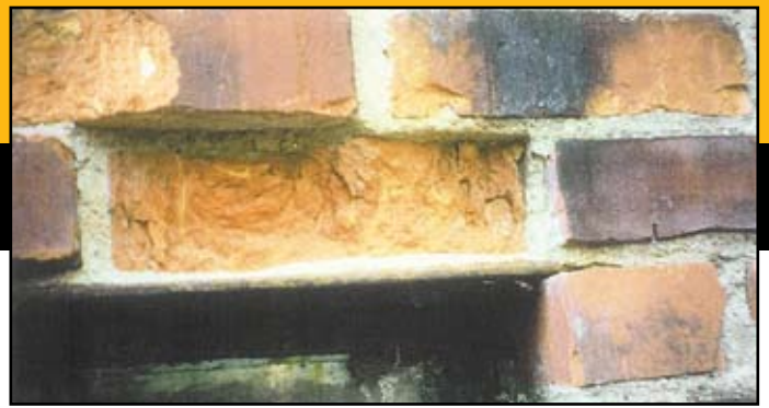
Close up of a typical exfoliated salmon face brick.
