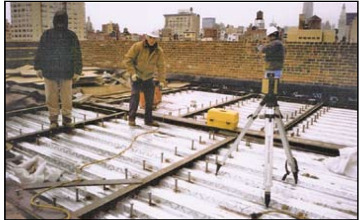
The new permanent metal deck and existing steel before pumping new concrete. The existing steel was cleaned and left in place. After removal of the existing slab, the temporary deck was removed and a new permanent deck (shown) was installed on new sister beams that are below the lines of the shear studs.
