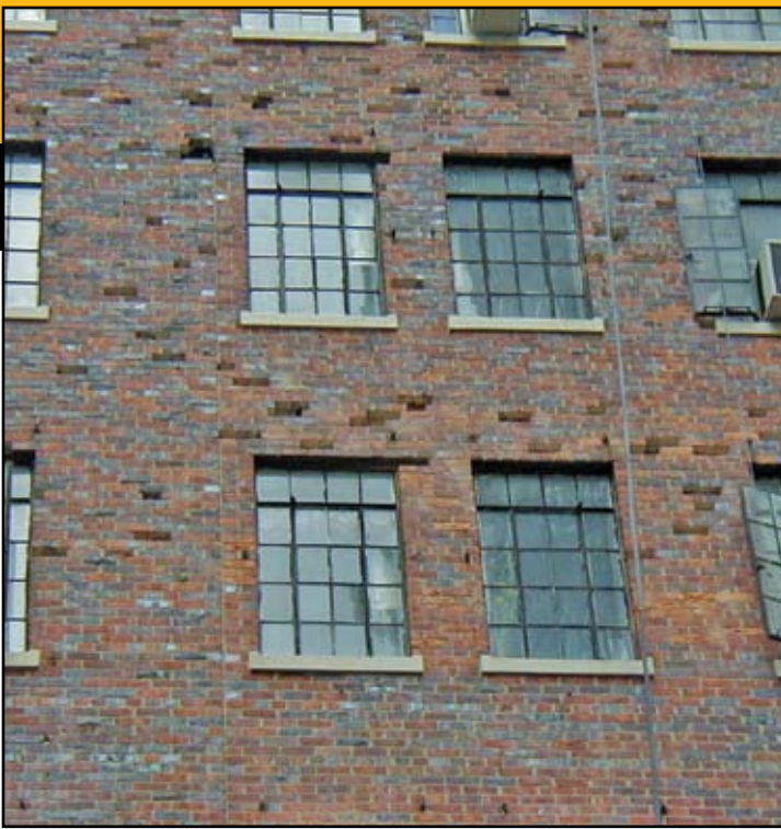
“Toothing” out of the exfoliated salmon (orange) face brick.
