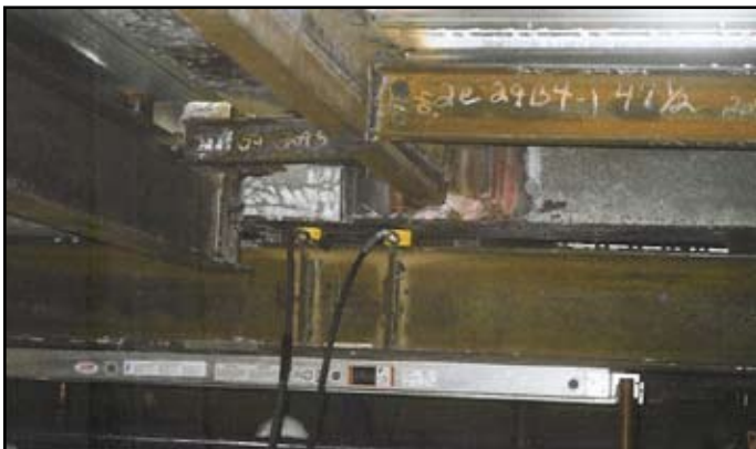
The existing concrete encased girder (top) being jacked against the new (lower) girder. Two calibrated jacks were used at each jacking location to permit the installation of a permanent bearing plate between them.
