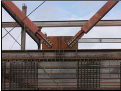
Connections between BRBFs and reinforced concrete shear walls required special seismic detailing.
