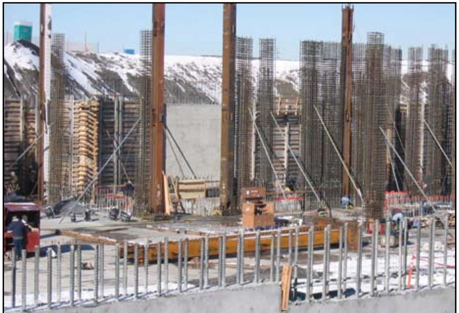
Integration of the large steel columns with the concrete shear walls required careful planning and coordination.
