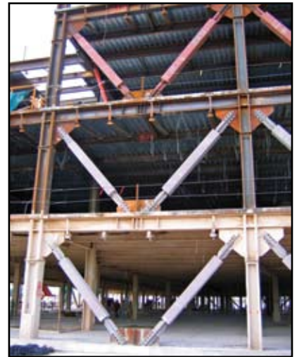
The configurations of the BRBFs are situated to work with the architect's layout of corridors, windows, stairs, and elevators.
