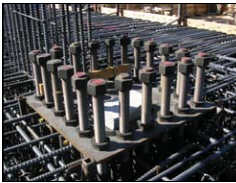
Anchor rods up to three inches in diameter were used to resist the tremendous uplift forces from the BRBF columns.
