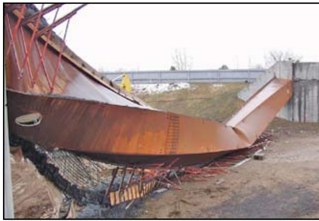
Figure 4: The Marcy Pedestrian Bridge following collapse during placement of the concrete deck.
