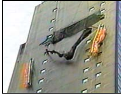
Figure 1: 540 Madison Avenue, partial facade collapse. Courtesy Channel 7 News.
