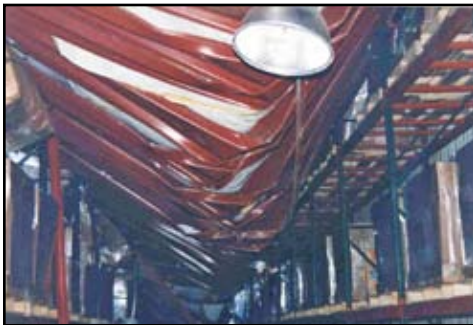
Figure 4: Rows of closely spaced Z purlins intended to carry the roof snow drift load rolled and buckled due to a lack of proper bracing as a result of a substantial number of missing purlin-to-roof connector clips
