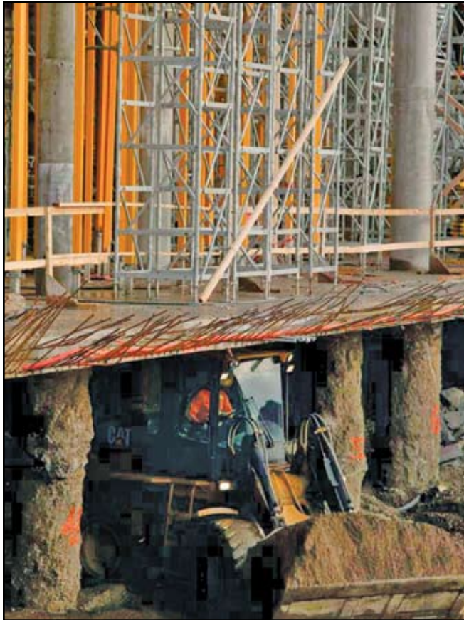
Figure 1: Excavation proceeds down to the P1 level while ground construction begins. (Photo by Pete Eckert)
