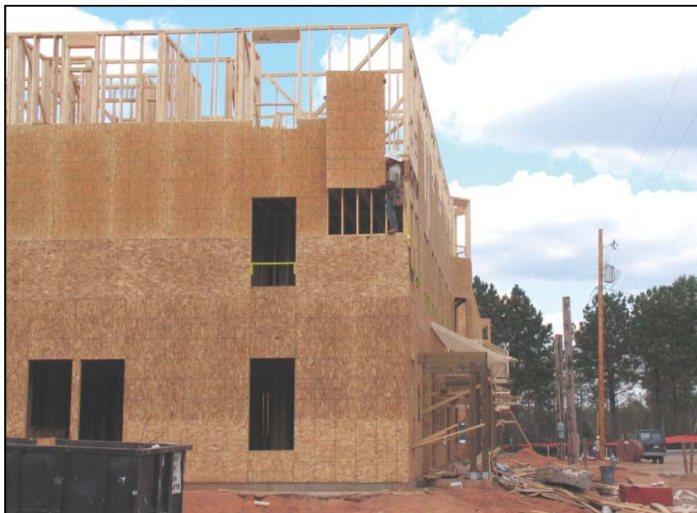
Framers install wood structural panel sheathing for vertical continuity to resist both shear and uplift in this multifamily project in Atlanta
