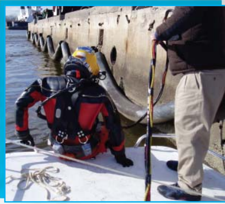
P.E. Commercial Diver entering the water to perform underwater investigation of a waterfront facility
