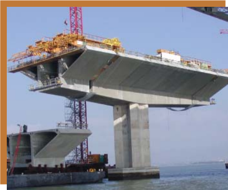
Figure 2: Segment Erection, San Francisco-Oakland East Bay Skyway Bridge Construction. Photo courtesy of Kiewit/Flatiron/Manson, A Joint Venture.
