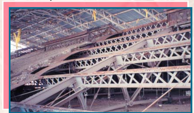
Roof section during construction showing temporary enclosures, framing and suspended interior platform
