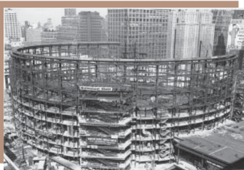
Madison Square Garden, New York City (1967). A photograph of Severud along with a model of the Garden's unique cable-supported roof was on the cover – and the feature story – of the June 9, 1966, issue of Engineering News-Record. Photo courtesy of Fred Severud, Jr.
