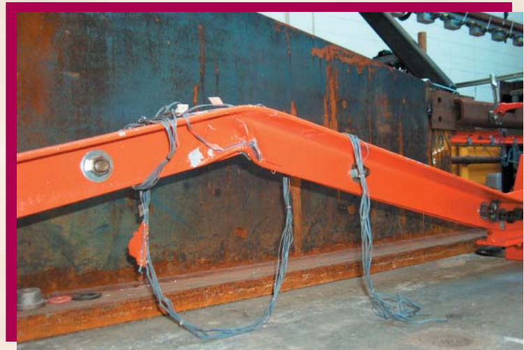
Figure 6: Local buckling at mid-span of double angle brace in compression
