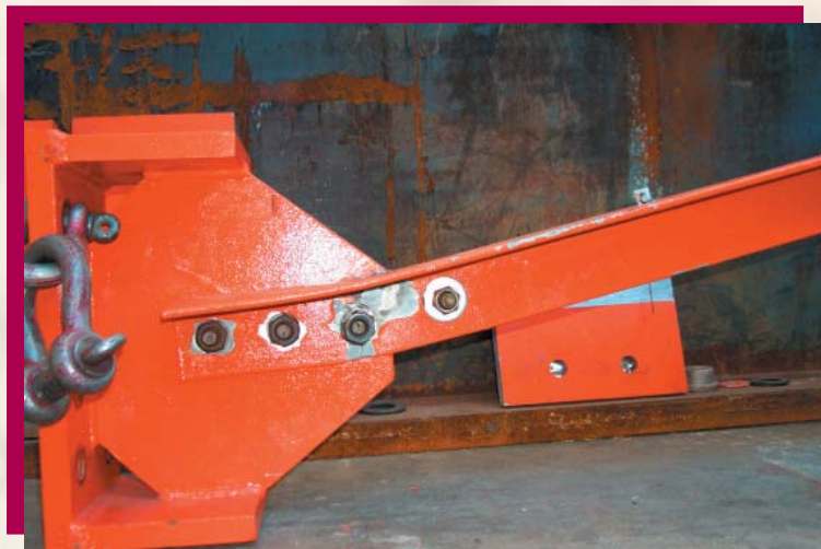
Figure 7: Fracturing of angle at point of plastic hinge development at brace end connection
