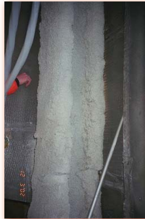
Figure 3: Structural Steel Column Protected with SFRM
