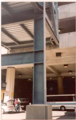
Figure 2: Steel Column Protected with Epoxy Based Intumescent (Photo Courtesy of PPG Industries, Inc.)
