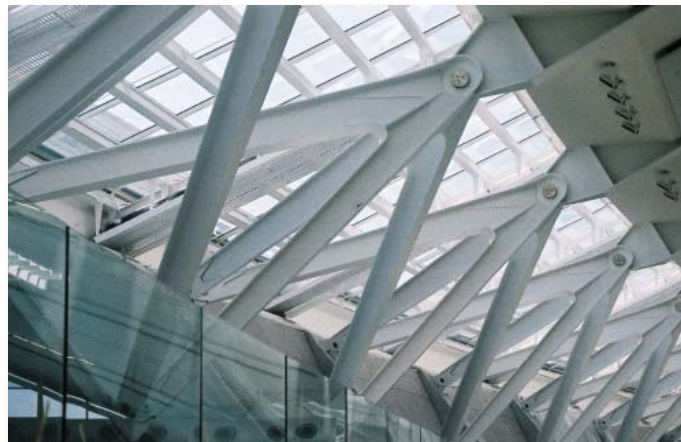
Figure 1: Structure Steel Members Protected with a Thin-Film Intumescent (Photo Courtesy of Isolatak International)
