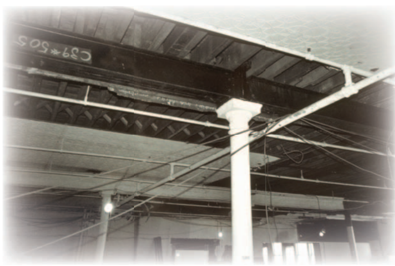
An interior cast iron column supporting a steel girder and wood joists.
