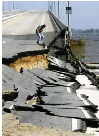
A Florida state bridge inspector looks at the destroyed bridge from Gulf Breeze, Florida to Pensacola Beach
