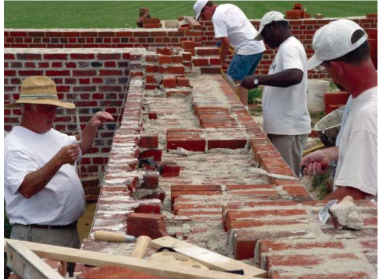
Using Traditional Lime Mortars in the reconstruction of the 17th Century Chapel at St. Mary's City, MD
