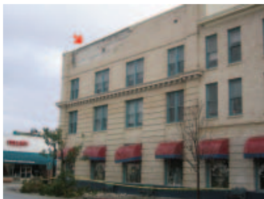
Figure 5 Masonry veneer peeled off the parapet of this building in Paso Robles
