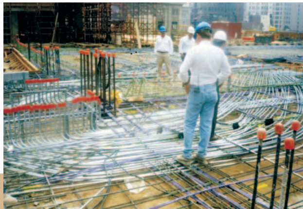
Not coordinating the conduit placement with the Electrical Engineer can cause a problem!
