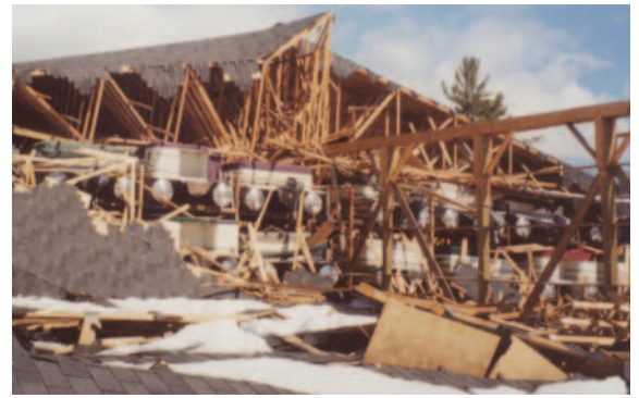
Photo: New England Winter Roof Failures; Courtesy of Pretzer Associates, Cranston, RI
