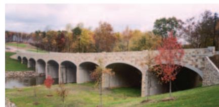
Largest installation to date (9 cell structure crosses 446-feet of the Goose Creek); Coton Bridge, Loudoun County, VA
